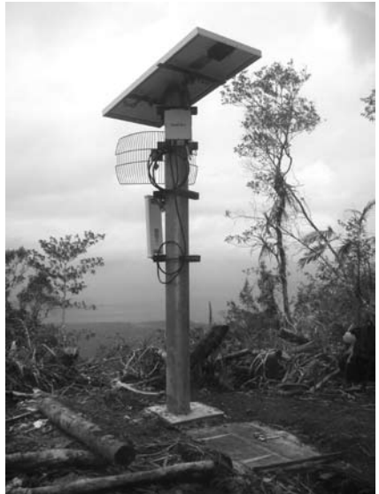
Solar-powered WiFi repeater station installed in the Solomon Islands.
